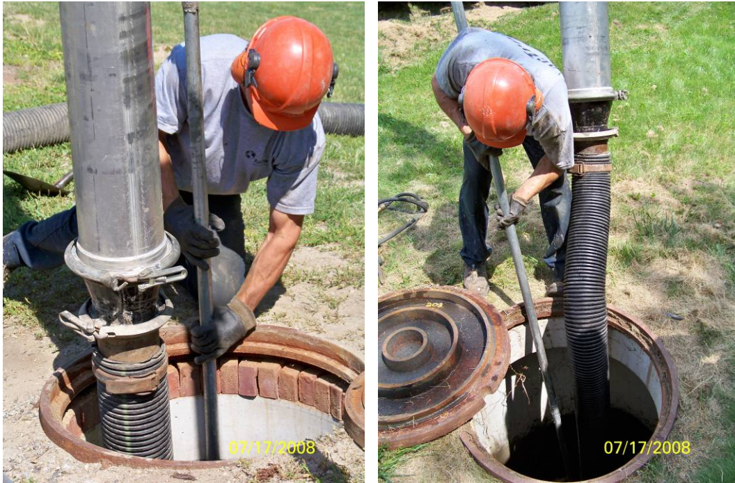
A maintenance worker stationed on the surface uses a vacuum hose to evacuate water, sediment, and debris from the system.
